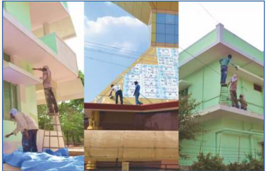
The Cosmic Tower has its golden coloured tiles worked upon. The Utility Block gets a fresh coat of paint after some repair work.
